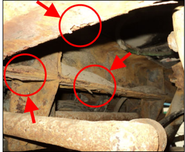
FIGURE 3: METAL FLAKING AND ACCUMULATED SAND
