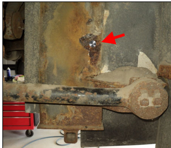
FIGURE 6: CLEANED SPOT ON STRUCTURAL MEMBER
