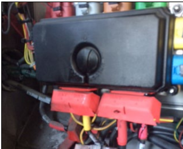
Rear Fuse Box, main power leads (12VD, 12VI, 24VD and 24VI)
