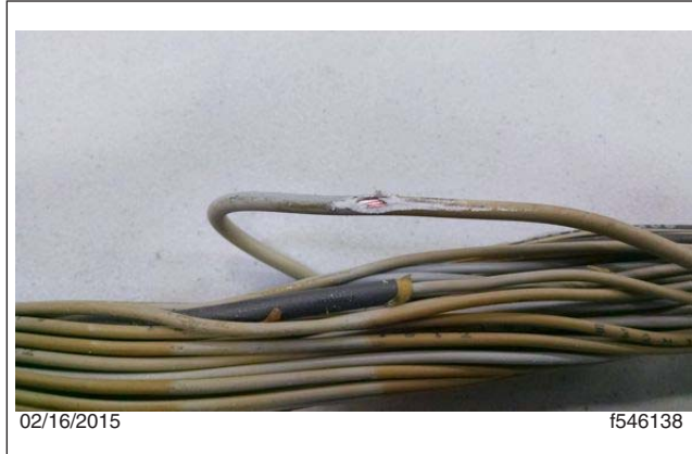
Fig. 1, Worn Insulation, Major
