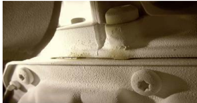
Figure 4. Leak located with talcum spray.
