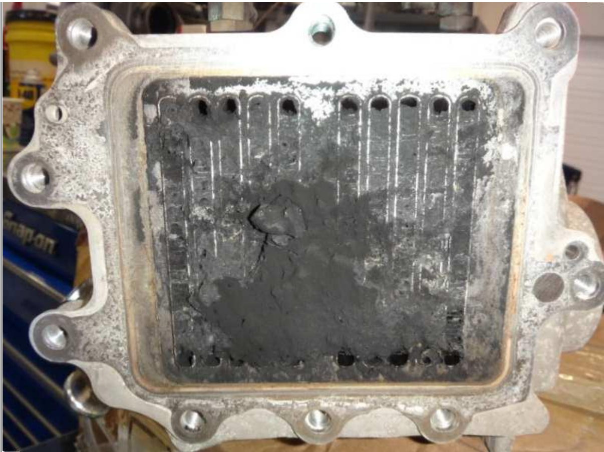
Figure 3: Soot Build-Up on the Core Face
