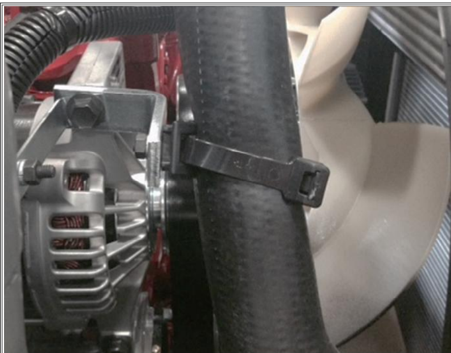
Figure 5: Issues – zip strap over tight, saddle clamp at incorrect angle, and extension bracket at incorrect angle causing saddle and strap to dig into hose
