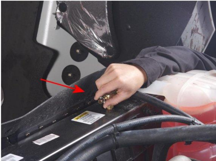
Figure 4 - Open air bleed on the top tank of the HTR
