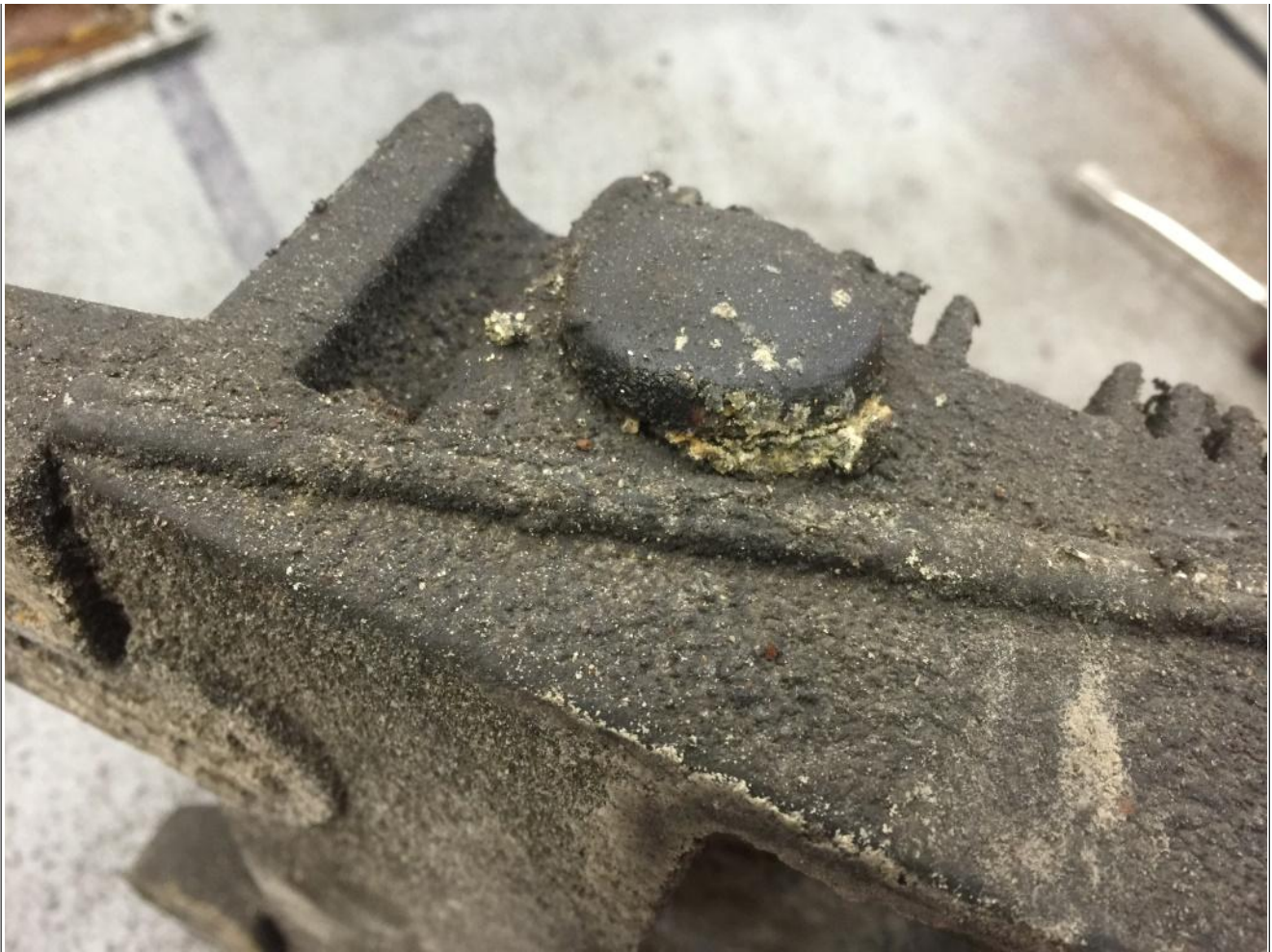
Figure 2: The plug is being pushed upward by debris and it is clear that debris has begun to enter inside of the housing. This RPM should be replaced.
