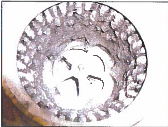
Figure 1. HV Battery Cooling Fan BEFORE Cleaning
