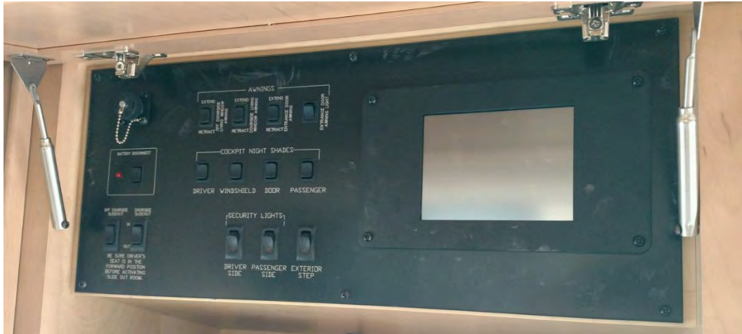
Picture: Front control panel
