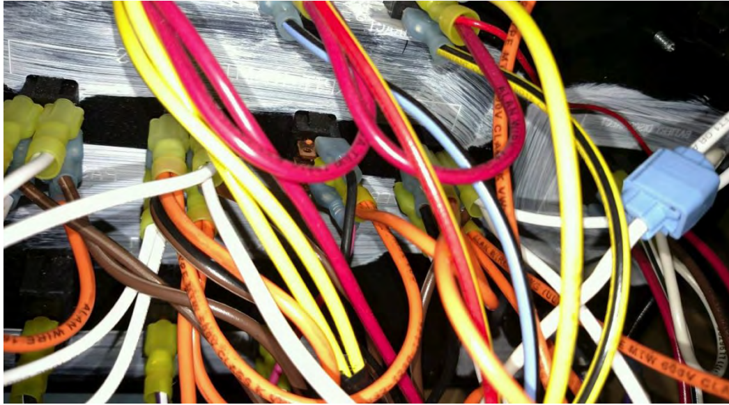
Picture: Control panel with complete wiring
