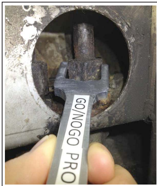
Figure 3 - Bulkhead Inspection with GO/NOGO Gauge N8902891
