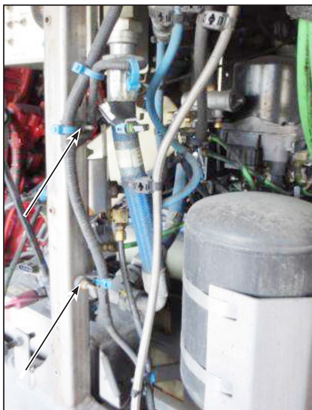
Figure 9 - Remove Electrical Harness from Structure
