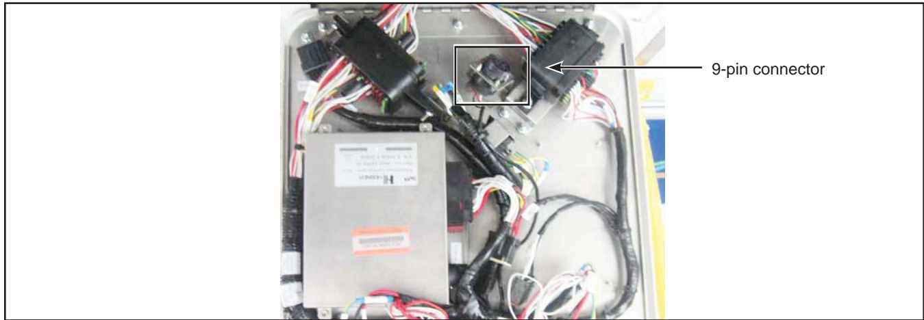
Figure 3 - ACU 9-pin Connector Location in RF9 Panel
