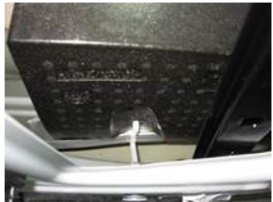
Figure 6. Zip tie cut.
