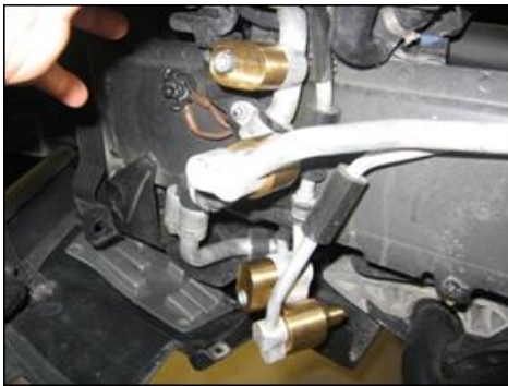
Figure 8. The location of the connections inside the left front wheelhouse on a Touareg with four zone climate control.
