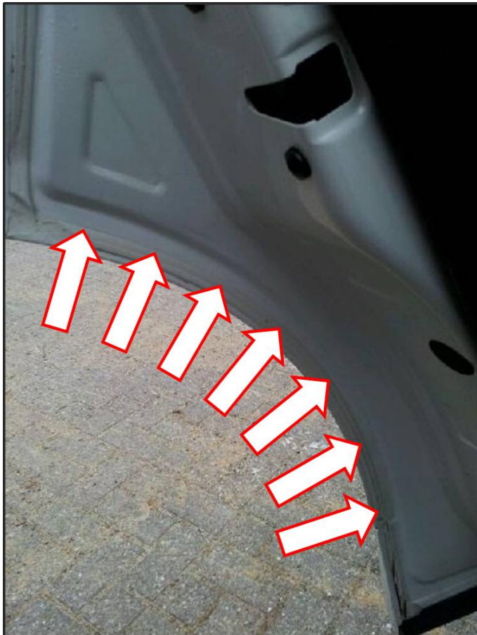
Figure 1) Arrows show the area affected by corrosion
