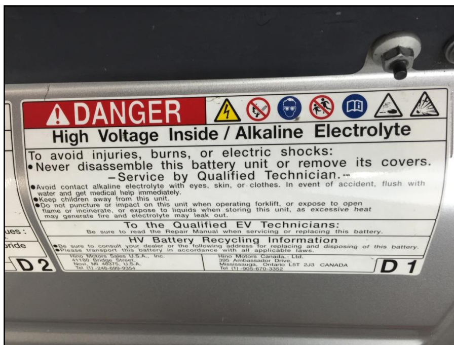
Red High Voltage Warning Label on Top of Battery Pack
