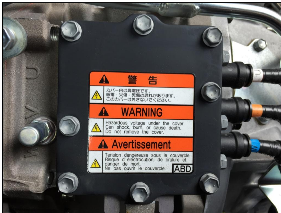
Orange High Voltage Warning Label on Motor/Generator Assembly
