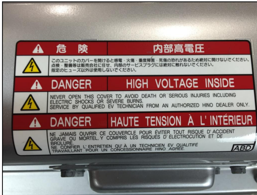
Red High Voltage Warning Label on Top of Battery Pack
