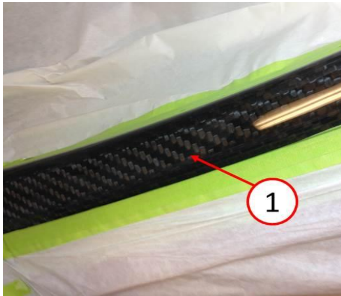
Fig. 7 Surface Condition Removed
