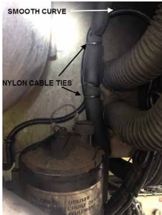
FIGURE 24 ROUTING BEHIND POWER STEERING RESERVOIR
