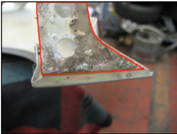
Figure 4 (corroded contact surface of fender)
