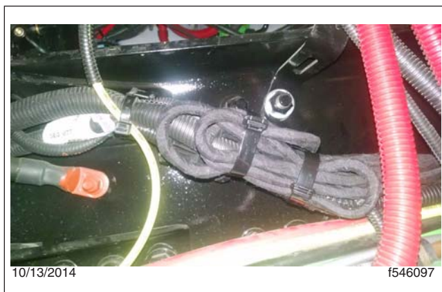
Fig. 5, Excess Harness Secured
