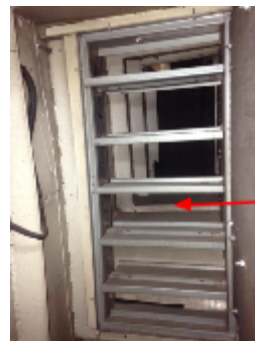
VIEW OF LOUVER IN THE OPEN POSITION Note: Missing seals on leading edge of vent louvers.
