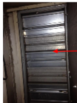
VIEW OF LOUVER IN THE CLOSED POSITION Note: Air can continually flow where seals are missing.
