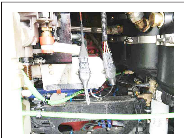
Figure 20 - Fire Suppression System Connectors
