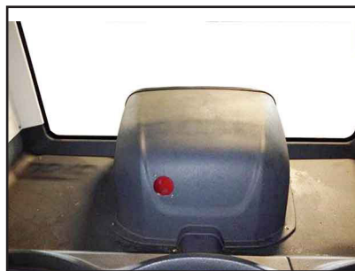
Figure 15 - Fire Suppression bottle Access Panel
