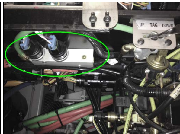
Fig.2 Switches and junction block
