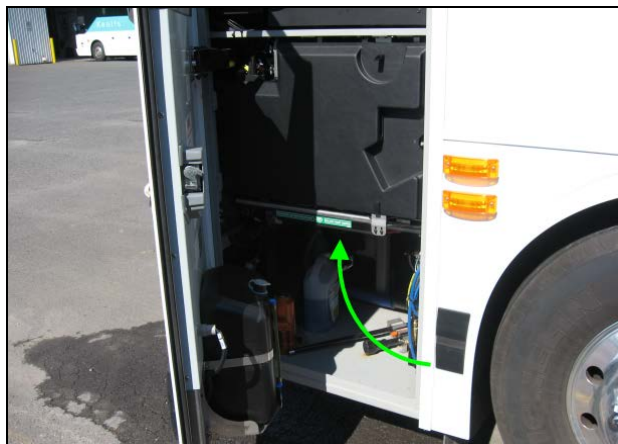
Fig.1 Pressure switches and module location
