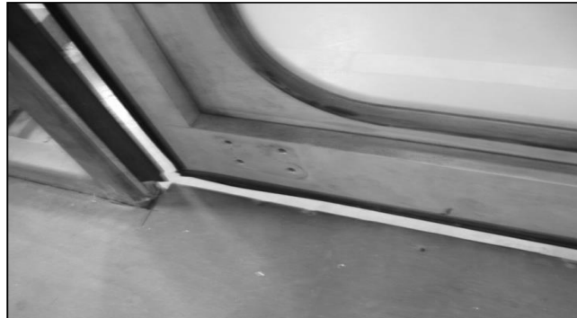
Figure 10 - Gap between Door and Jamb Seals Prior to Final Adjustment
