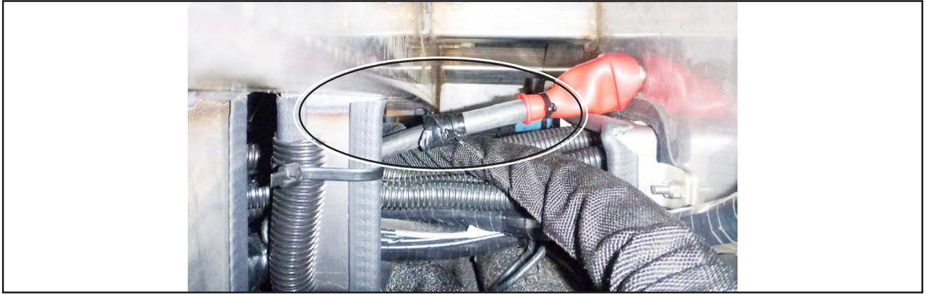
Figure 30 - Power Cable Routing
