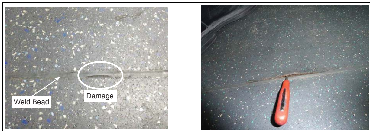
Figure 1 - Left Picture: Damaged Weld Bead Section on an Undamaged Floor Covering (Level 1: Repair) Right Picture: Damaged Floor Covering (Level 2: Replace)
