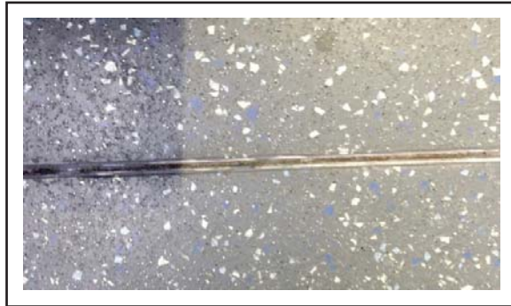
Figure 3 - Damaged Weld Bead Removed
