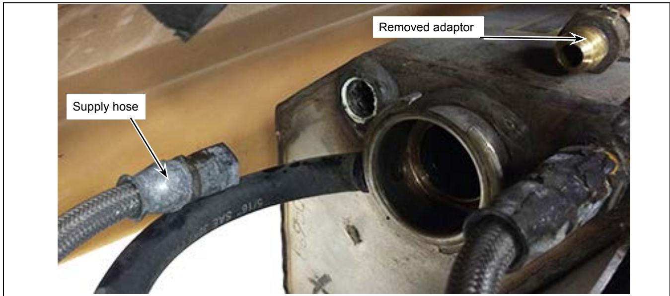
Figure 3 - Supply Hose Linking the Surge Tank and the Radiator Collector
