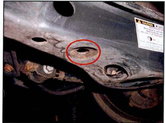
Figure 2. Stabilizer Link Damaged
