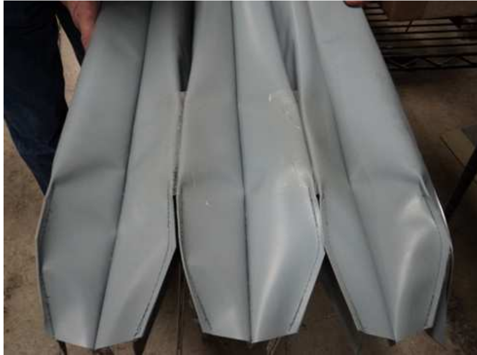
Figure 4: FALSE CEILING BELLOWS REPAIR (TAPE HOLDING FOLDS TOGETHER)
