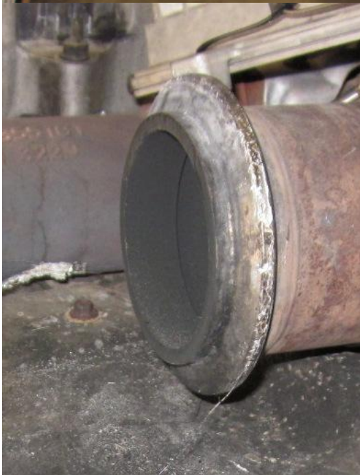
Joint & Clamp Location at Rear of Engine
