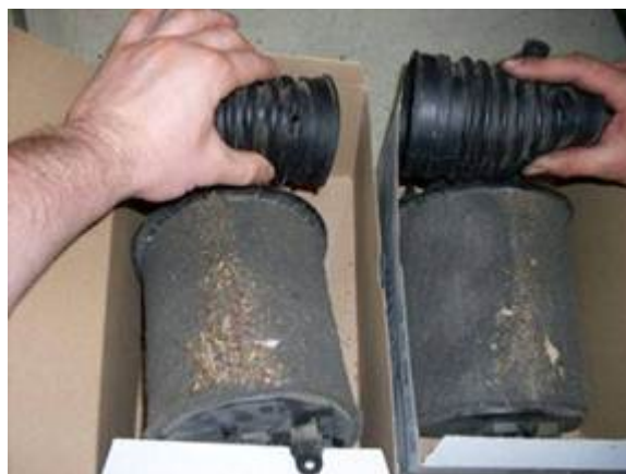
Figure 1. Example of excessive dirt on air filters.
