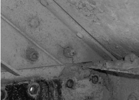
Figure 7: crack on side extrusion.
