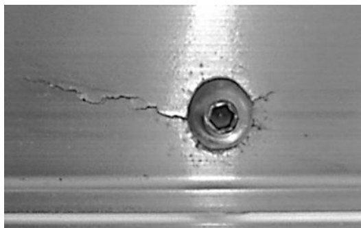
Figure 4: Spider crack on bottom rail
