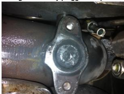
Figure 3 – Fully plugged AFI port
