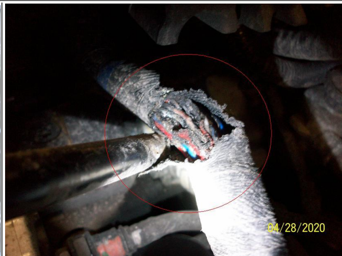
Photo 2 - Example harness and wire damage
