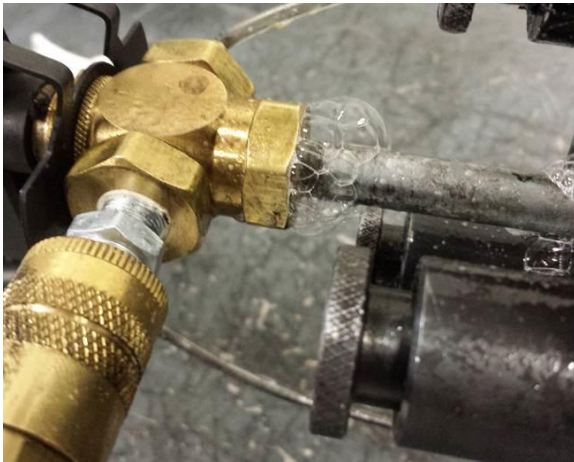
Figure 4: Air fitting leaking at "T" connector
