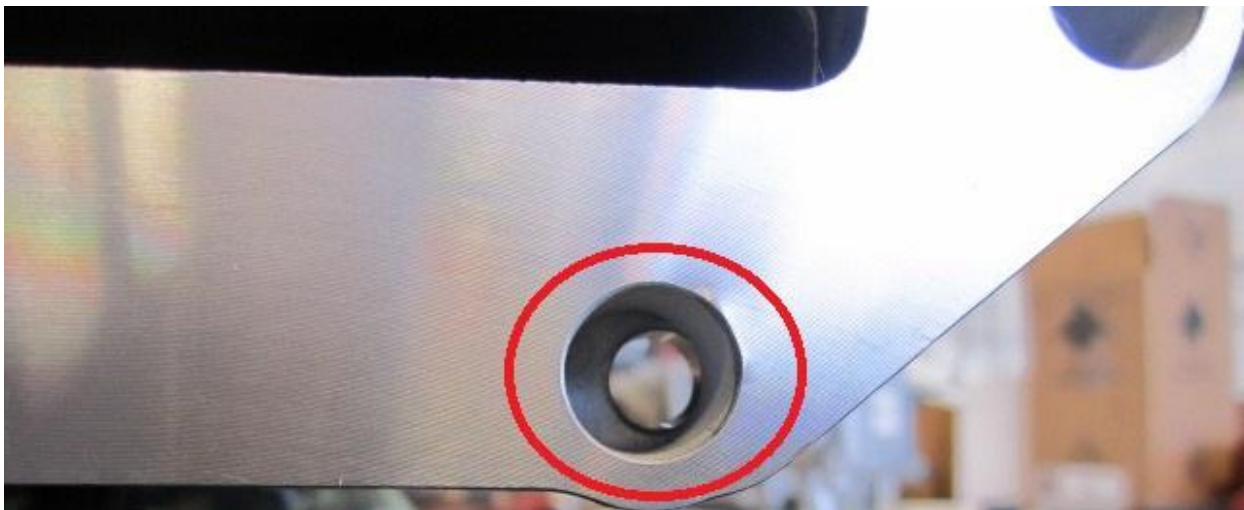
Red circle is the area of concern
