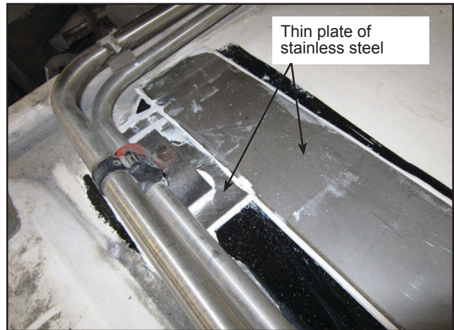
Figure 6 - Severe Damage Repaired with a Stainless Steel Plate.
