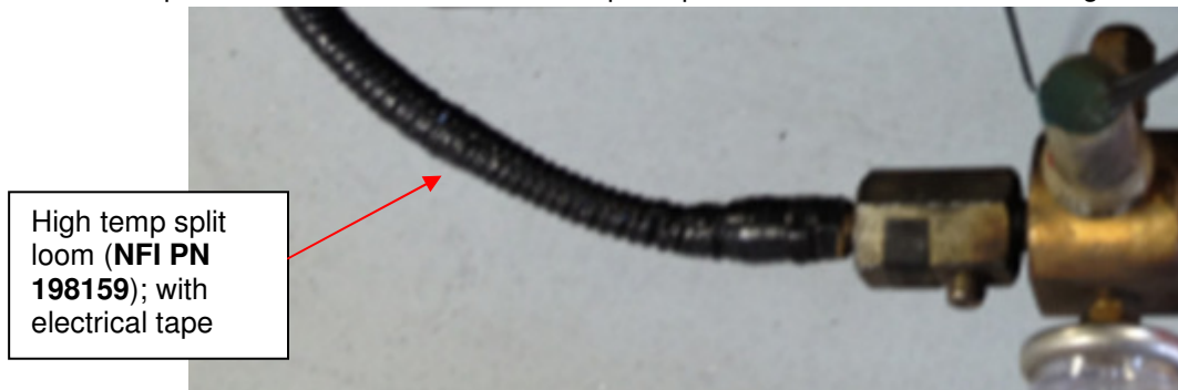
Fig 8 – Fire suppression hose with loom and tape
