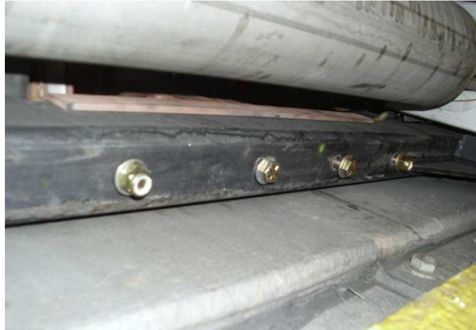
Figure 29: Generator mount hardware
