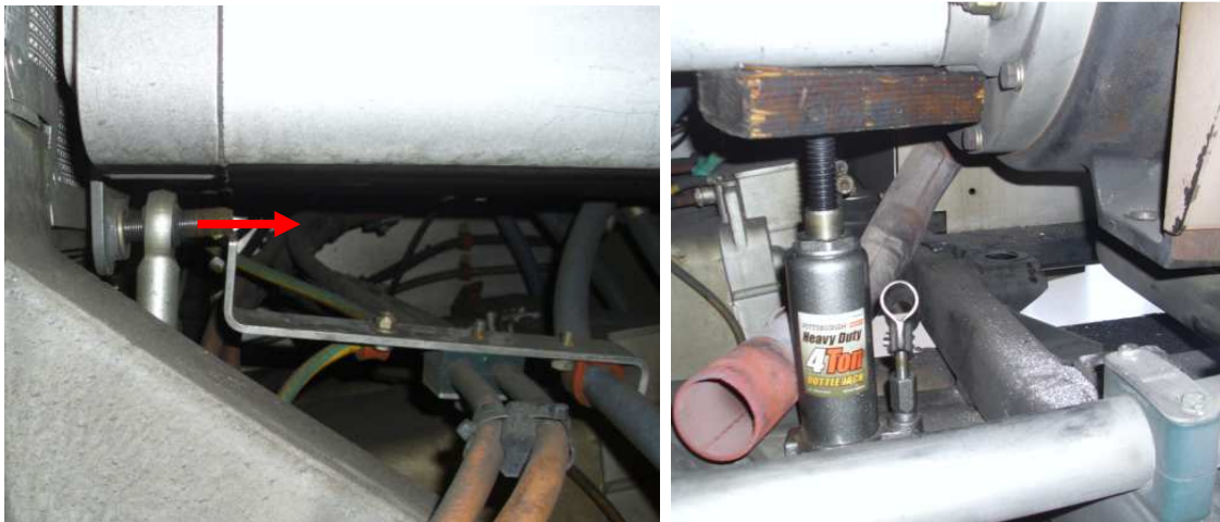
Figure 11: Generator Mount Support
