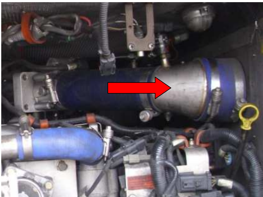
Figure 40: Installed Air Intake
