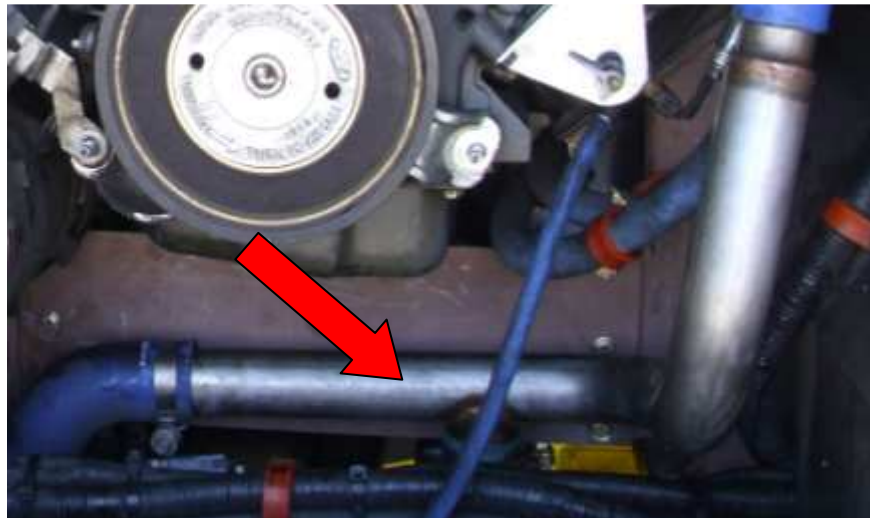
Figure 38: Installed Coolant Tube
