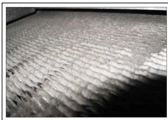
Figure 10 - Dirt on Evaporator Coil
