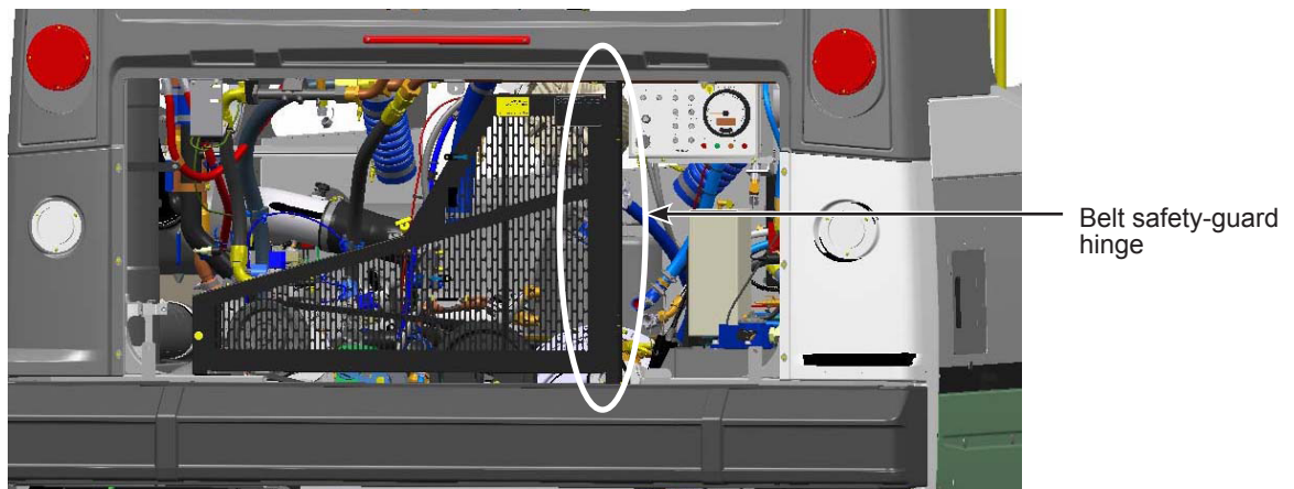
Figure 1 - Belt Guard Location
