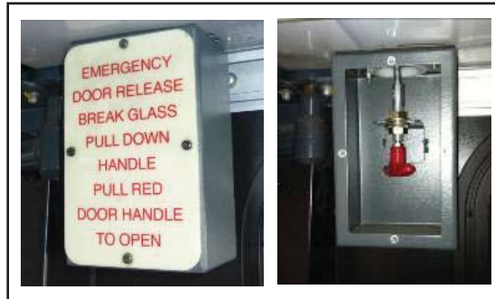
Figure 5 - Emergency Door Release Cable Box Front Plate Removal
