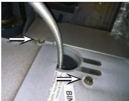
Figure 6 - Emergency Door Release Cable Box Bolts
