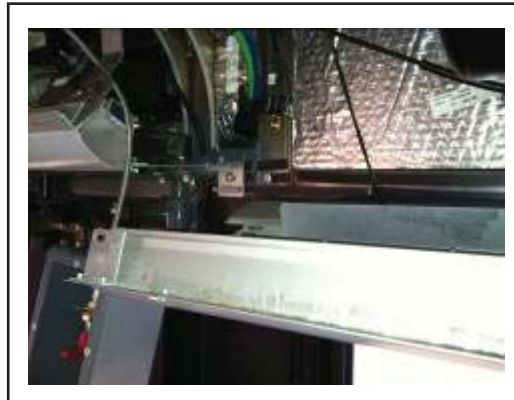
Figure 11 - Broken Panel Removed
