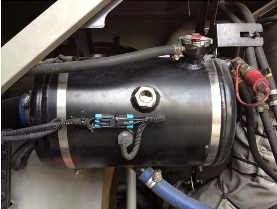
NEW COOLANT SURGE COOLANT SURGE TANK INSTALLED
