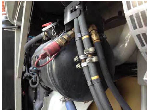
NEW COOLANT SURGE COOLANT SURGE TANK INSTALLED - CURB SIDE
