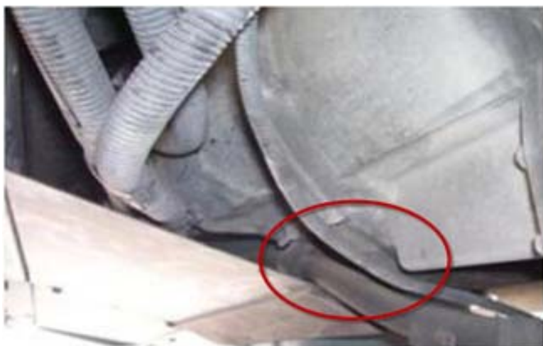
Figure 3 Evidence of Transmission Cooler Hose Abrasion
