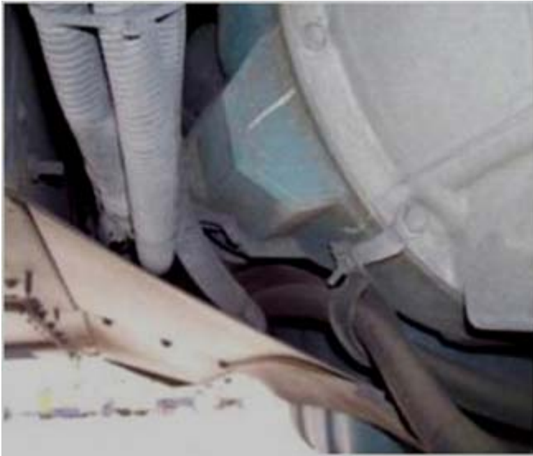
Figure 4 Areas Accessible from under the Unit Looking into the Air Management Panel Area
