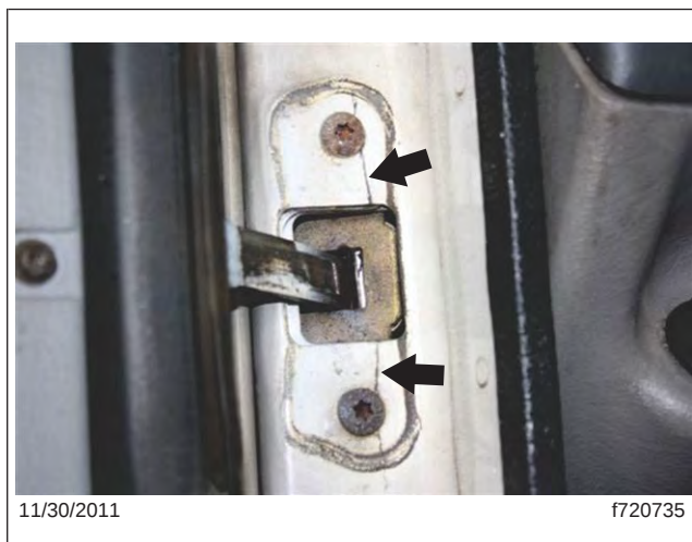
Fig. 1, Example of Door Frame Cracking
