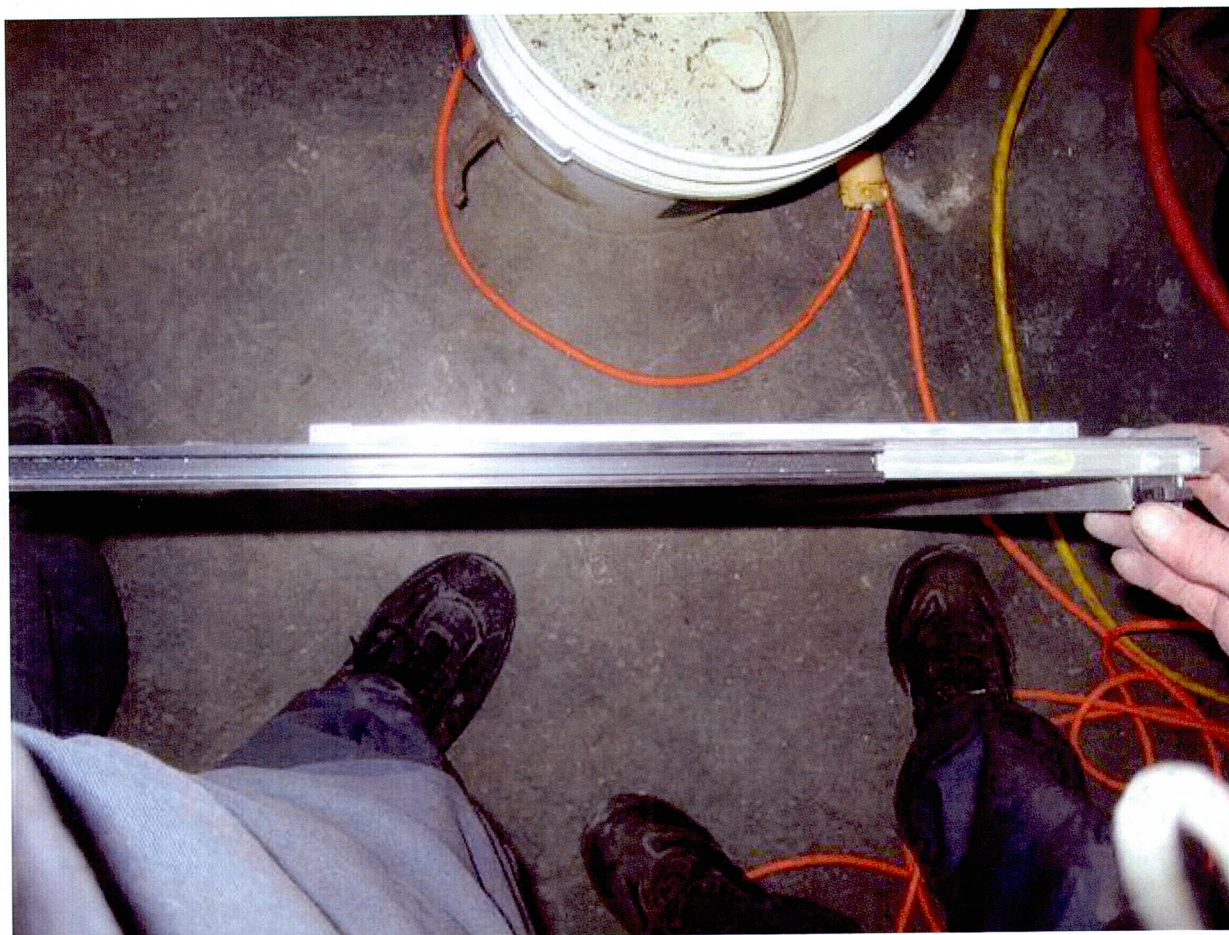
Above photo shows the plastic guide loose and out of position.
