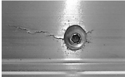
Figure 4: Spider crack on bottom rail
