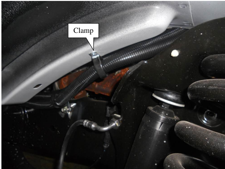
Practice 7: Where cables must run through difficult areas like this wheel well, use p-clamps to secure them in one spot.
