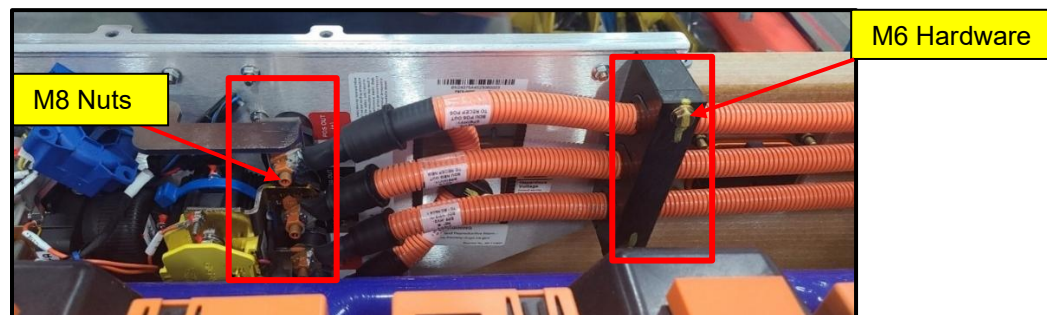
Figure 6: High Voltage Cables on BDU
